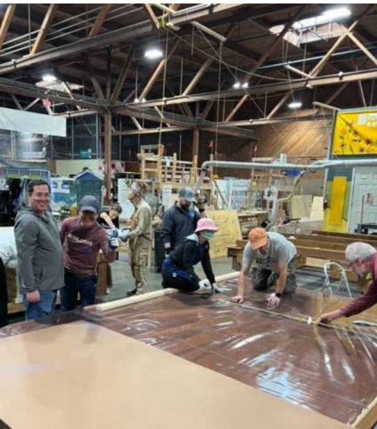
Executive Committee members Seth Millstein, Evan Brown, Will Young, and Erin Varriano were among those who helped build wall sections for Sound Foundation tiny houses at the Section volunteer event in September.
